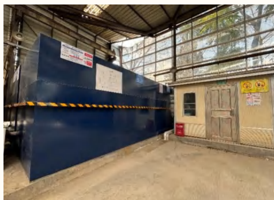
Sewage Treatment Stations
